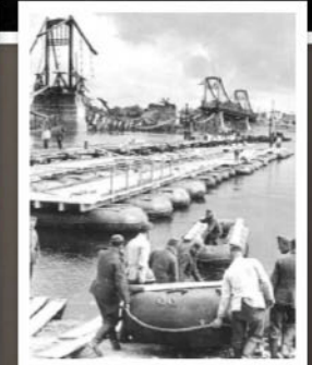
Above: German engineers build a pontoon bridge over the Dniepr River at Kiev in less than a day
